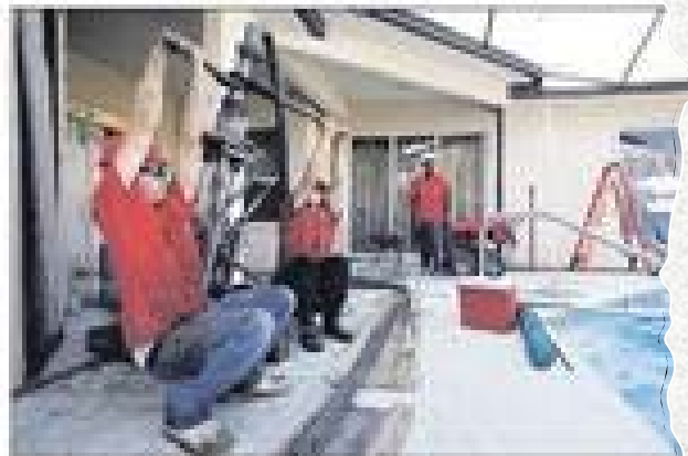
After Hurricane Ian, an interior foundation crack widened to a hole and pouring concrete into the hole. The hole was about 2 feet wide and 1 foot deep. Photo by Tommie Williams for the Tampa Bay Times.
